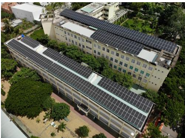
Figure 2: Rooftop solar power project (phase II)
