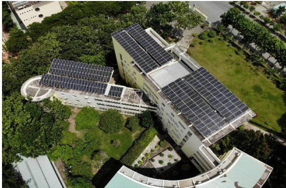
Figure 1: Rooftop solar power project (phase I)
