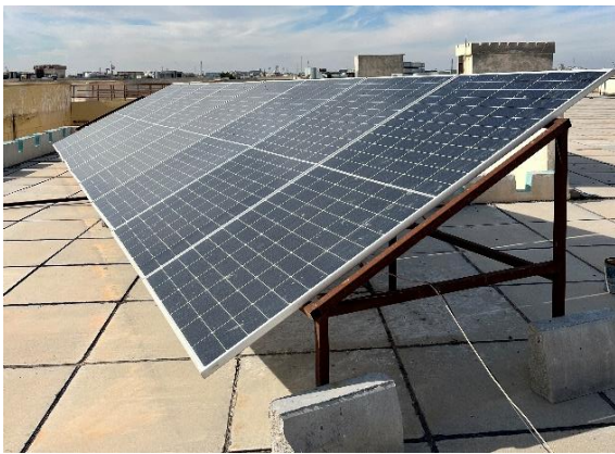
Figure 4. Solar panels array setup
